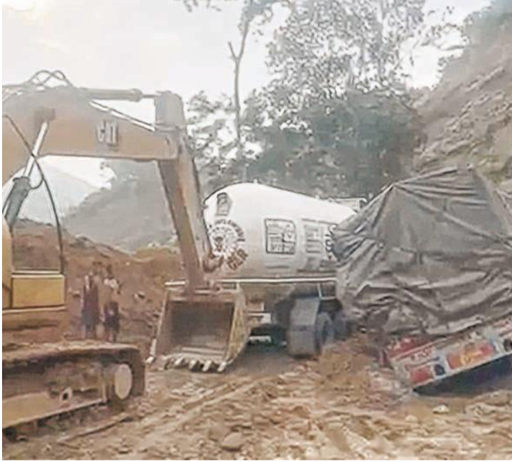
road damage along the highway, leaving hundreds of vehicles,
